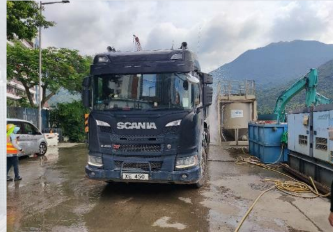
Wheel washing facility at the site exit
